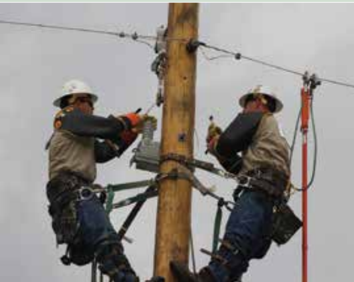
Left to Right: CCECI Apprentice Linemen Justin Hubert and Jacob Haselhorst can be seen here performing a single phase capacitor changeout.
