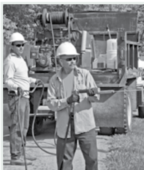
Mechanic Ron Deien and Field Serviceman Dale Nordike continue spraying powerline rights of way throughout the summer. The spraying helps prevent costly tree trimming as well as nuisance outages due to overgrown trees growing into the powerlines.
