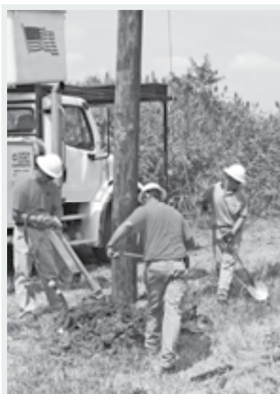
Foreman Doug Vonder Haar and Apprentice Linemen Adam Robke and Mike Faust tamp fresh dirt around a new pole that has been set. They have been doing extensive upgrades to some older lines near the Shattuck area over the past several weeks.
