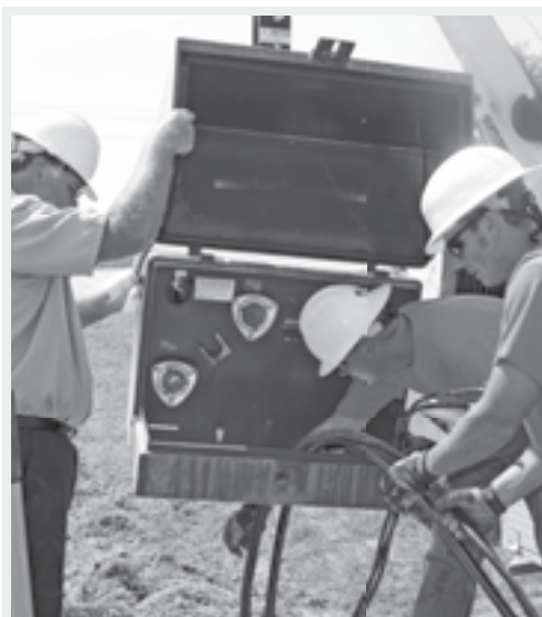
Foreman Gary Albers and Apprentice Linemen Craig Benhoff and Tyler Koerkenmeier install a pad mounted transformer near Carlyle. More than 85% of the new services installed on CCEC's system are fed by underground cables and equipment.
